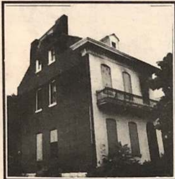
This building at 1713 S. 7th caught fire three times before it was damaged enough to be razed.
