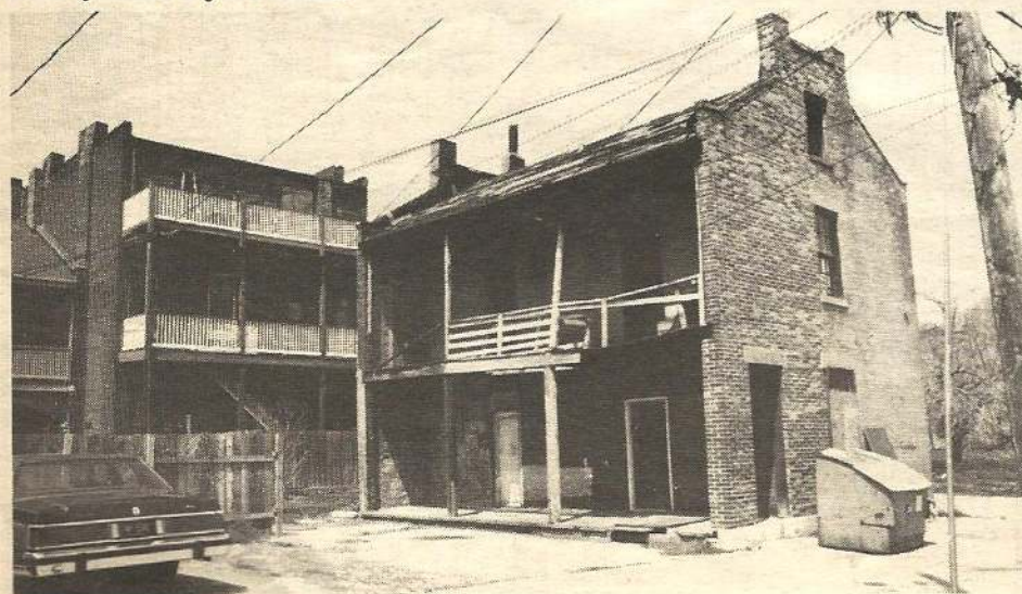
Sagging rear end.
