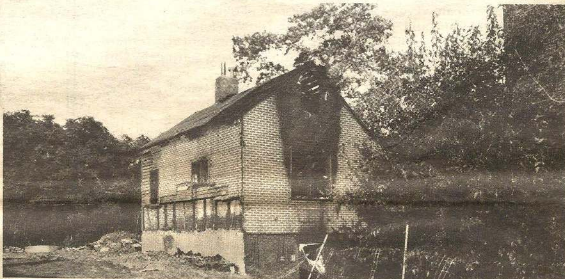
This fire-damaged cottage may be the oldest extant structure in the City of Saint Louis.
