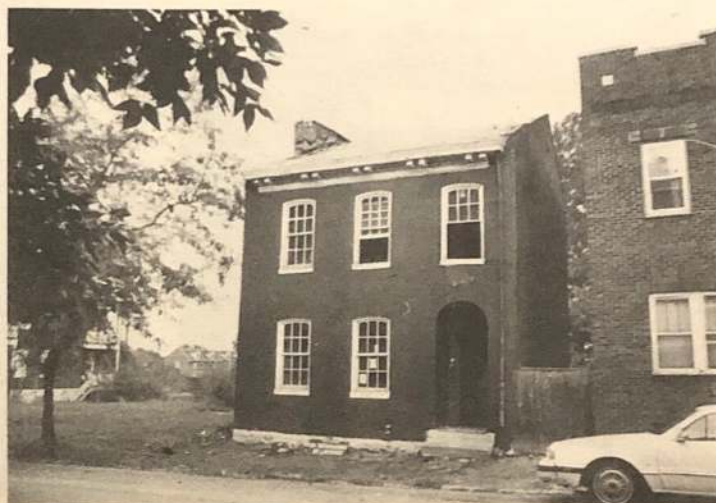
2350 Menard as rehab was beginning. Tarps form a temporary roof.
