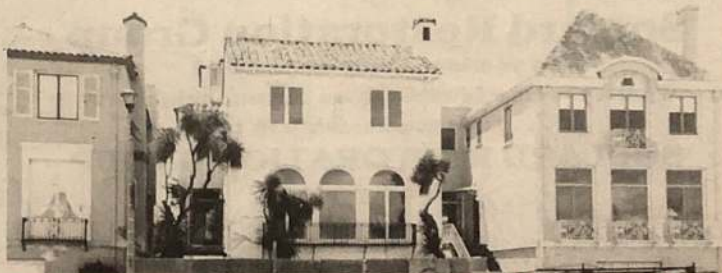
The structural cracks are clearly visible on this San Francisco townhouse, damaged in the 1989 Loma Prieta earthquake. How well Souldard's buildings will survive an earthquake depends on a number of factors, not the least of which is how well you prepare for the eventuality.
