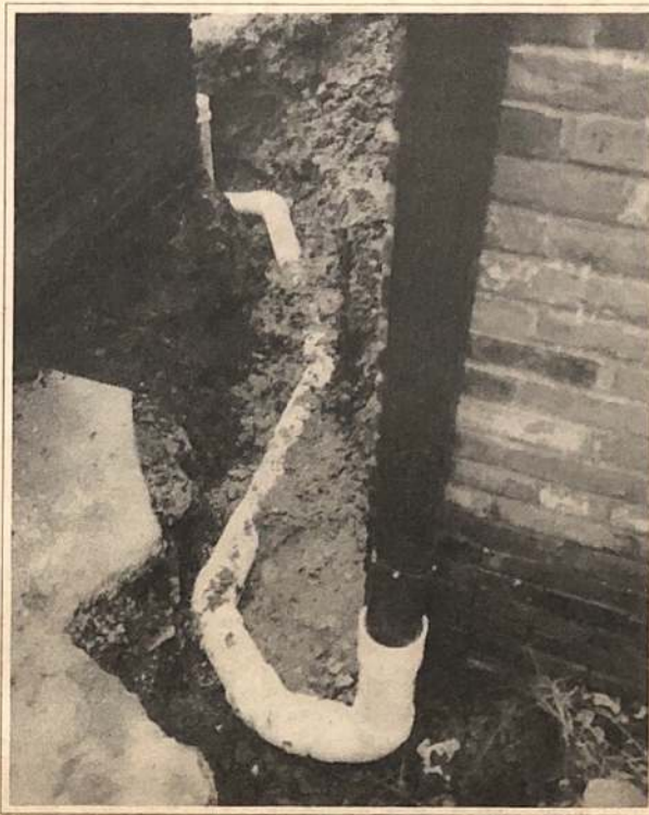
An infamous downspout—connected at last!
